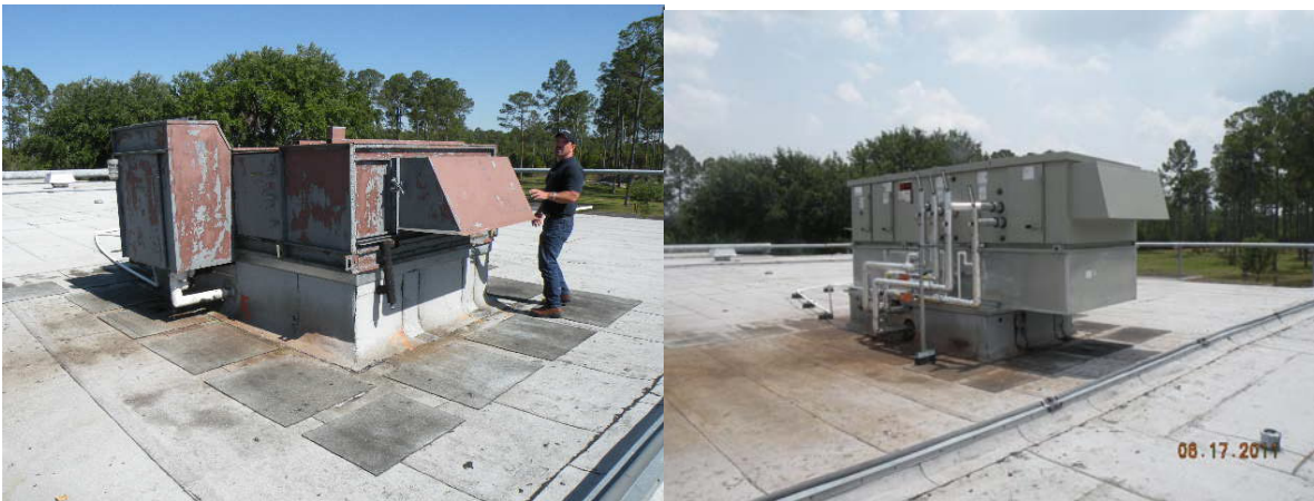
Air Handling Unit at Northeast Florida State Hospital (Macclenny) replaced with fixed capital outlay funding
