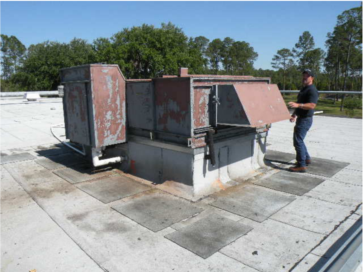
Air Handling Unit prioritized for replacement at Northeast Florida State Hospital (Macclenny)
