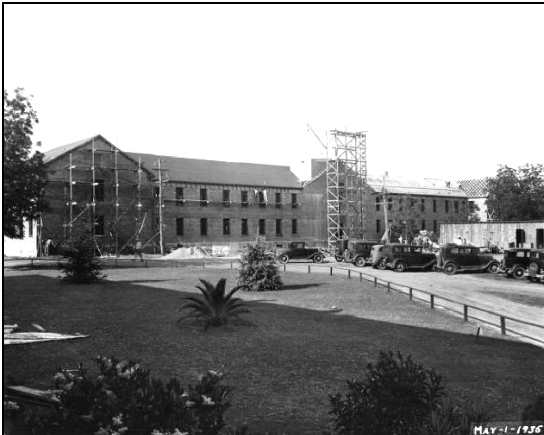
A 1936 building construction project at Florida State Hospital (Chattahoochee), funded by W.P.A.
